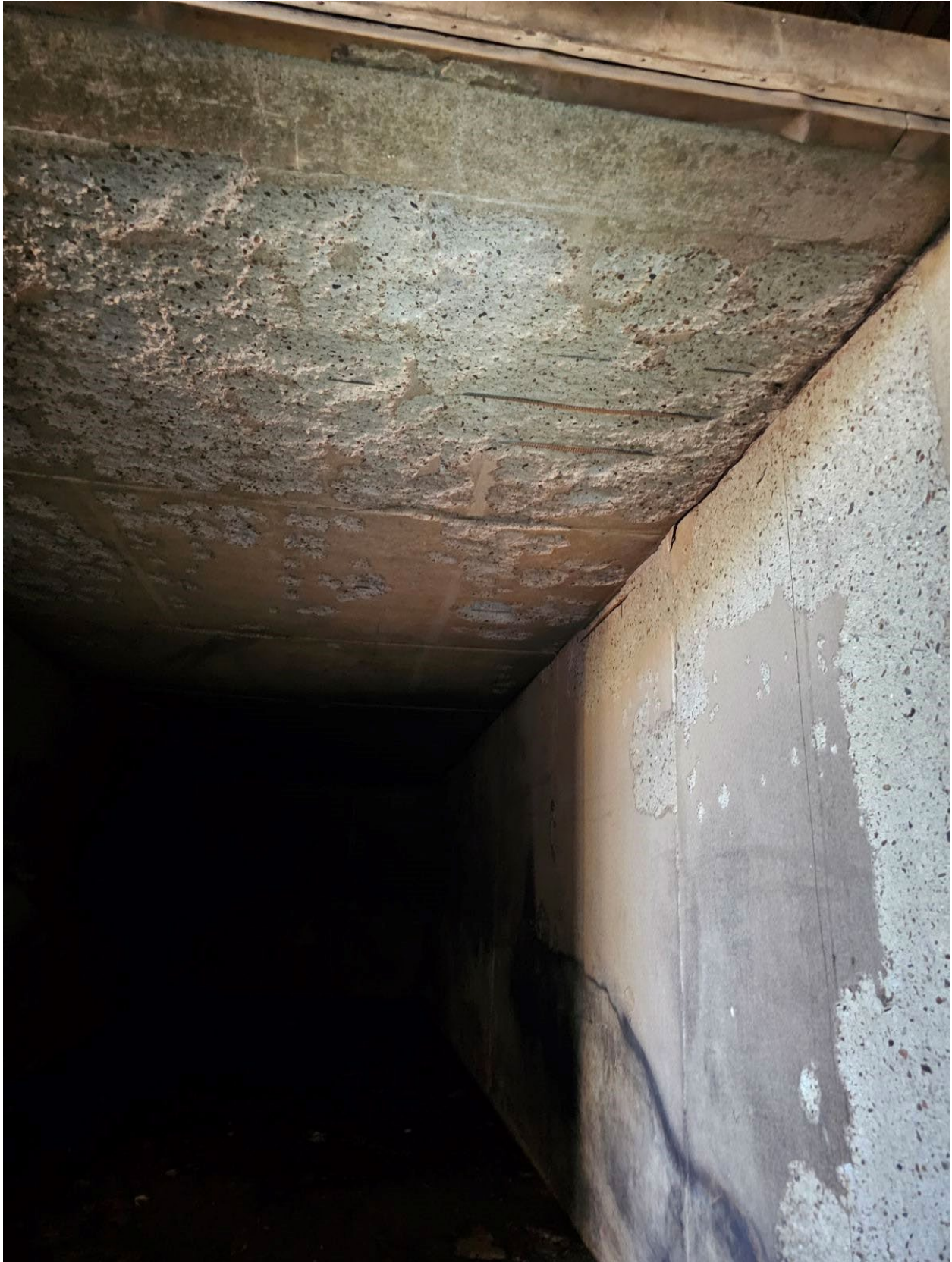
Figure 3: Damaged Concrete and Exposed Rebar - Vault #3
