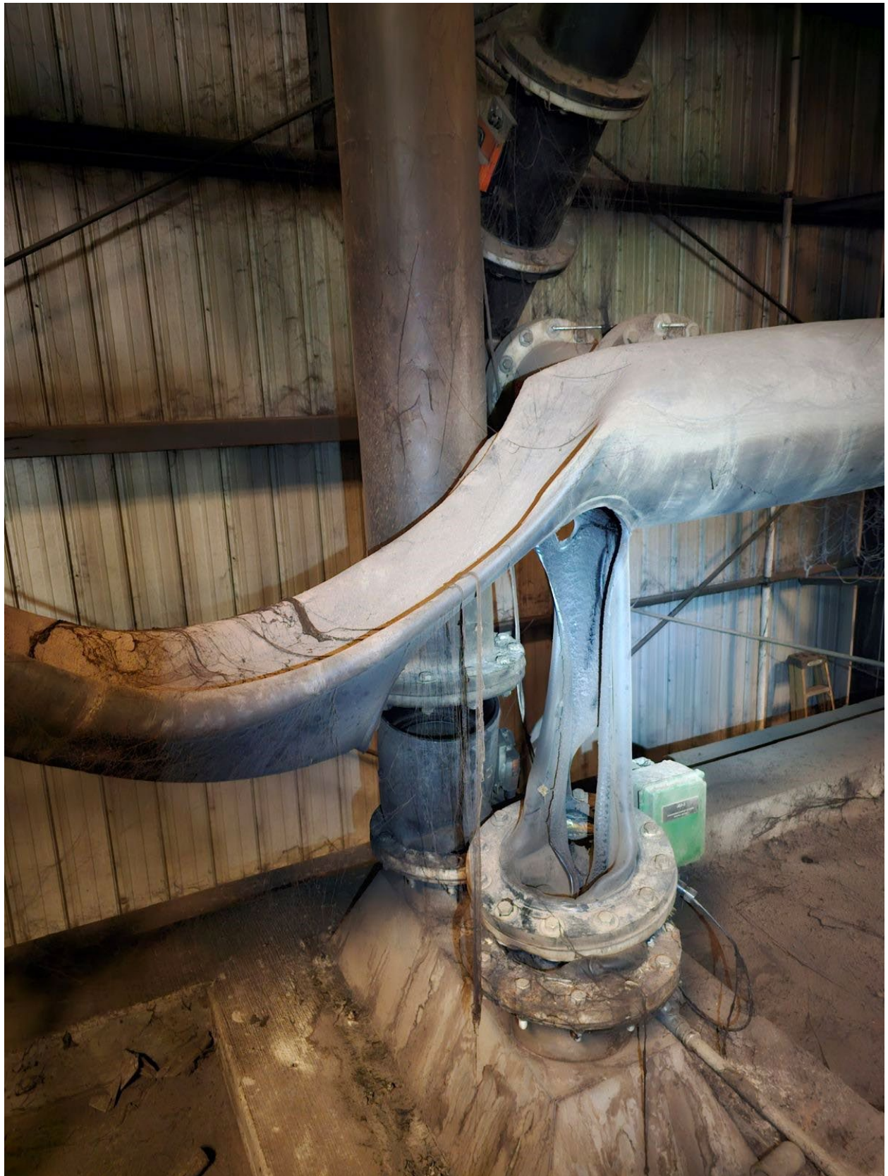
Figure 4: Melted Ventilation Pipe on Vault Roof
