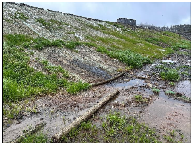
Figure 62 - Leachate near toe of slope.
