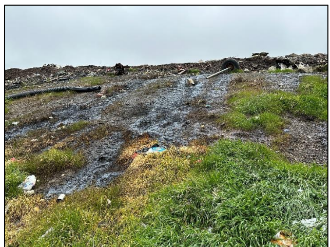
Figure 65 - Leachate seeping at top of slope.
