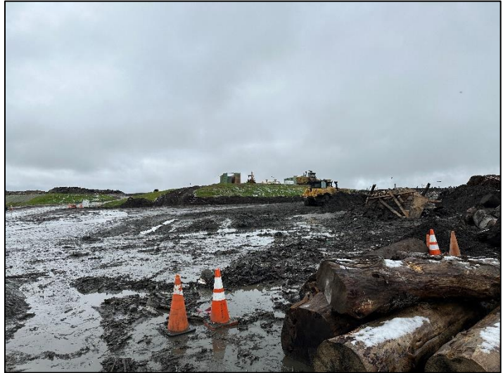
Figure 42 - Ponding on landfill at C&D and wood area.
