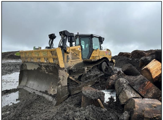
Figure 4 - Dozer parked in ponded stormwater.
