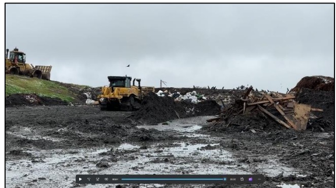
Figure 40 - Ponding at landfill tipping pad.
