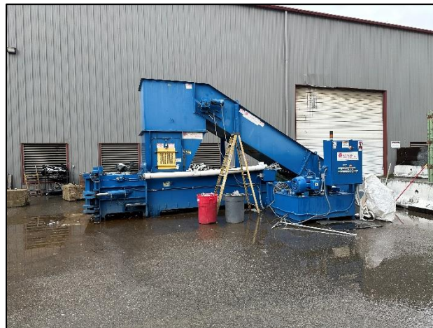
Figure 72 - Baler at the main transfer station.
