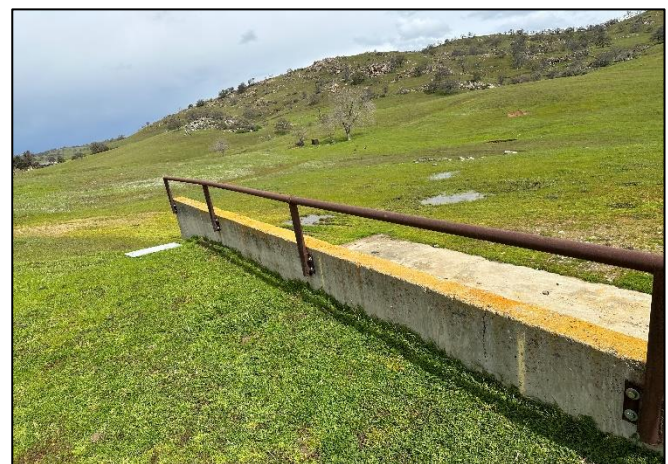
Figure 20 - Hornitos Container Site - Rail
