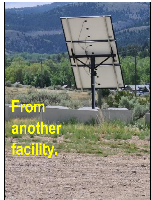
Figure 27 - Solar Panels - Madison County, MT
