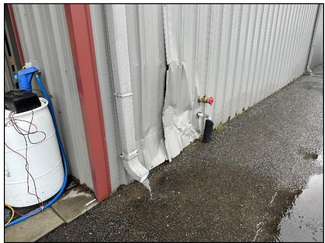
Figure 38 - minor building damage - repair as needed.
