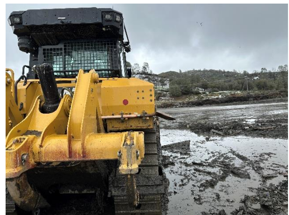
Figure 32 - Poor grading on top of landfill.
