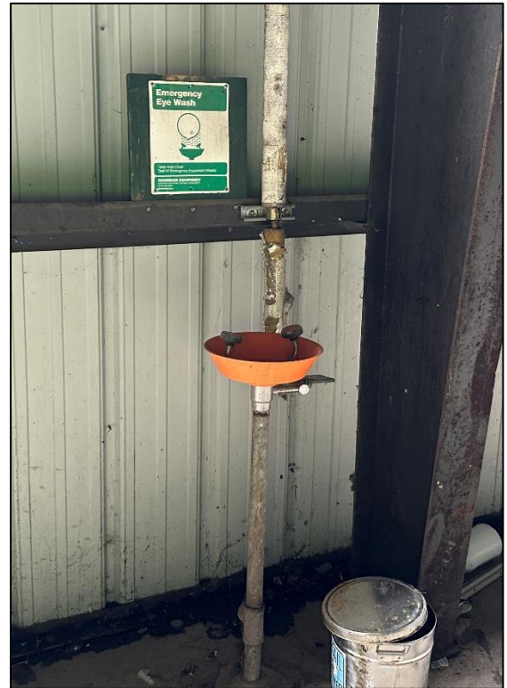
Figure 73 – Cal/OSHA-required eye-wash station does not work.
