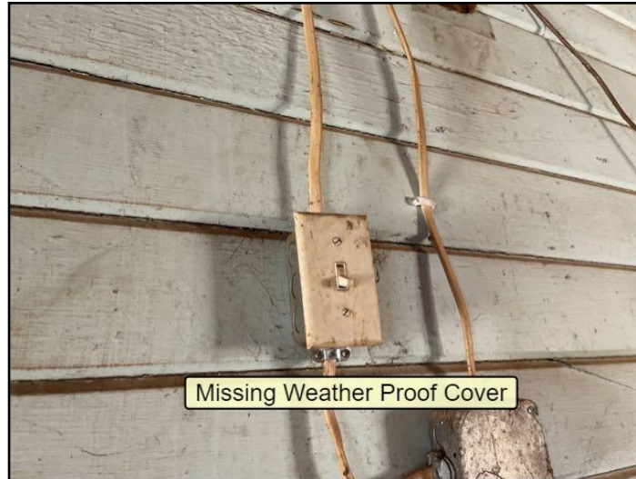
43. Missing Weather Proof Cover
