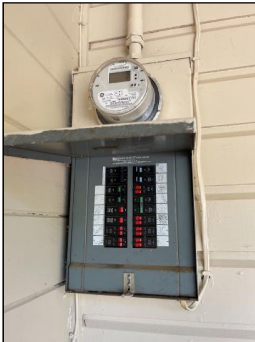
31. Breakers - exterior wall
