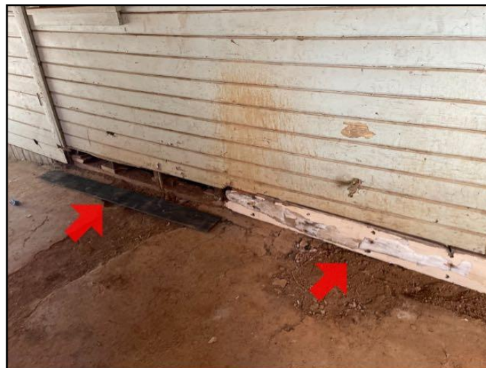
19. Siding is not installed.
