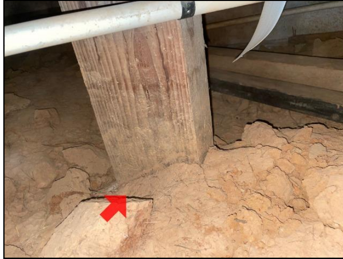
25. Earth To Wood Contact. Recommend checking...
