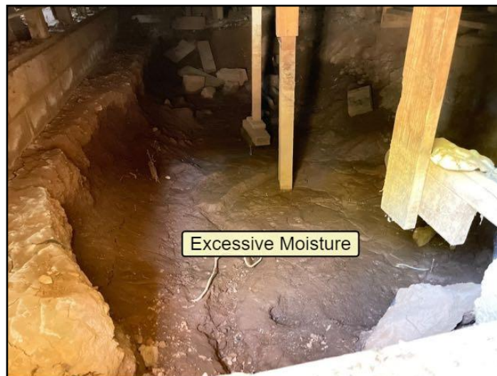
24. Excessive Ground Moisture
