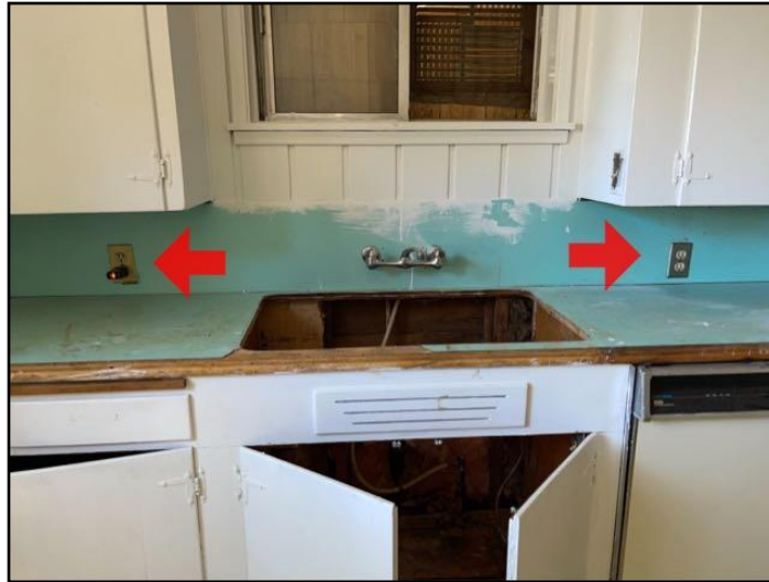
39. Ground needed for 3-slot outlet
