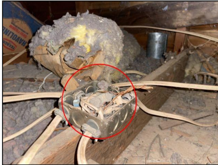
37. Cover loose or missing
