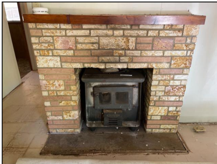
49. Wood-burning fireplace - not in service
