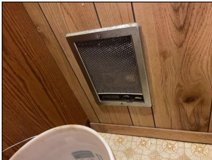
48. Electric Wall Heater
