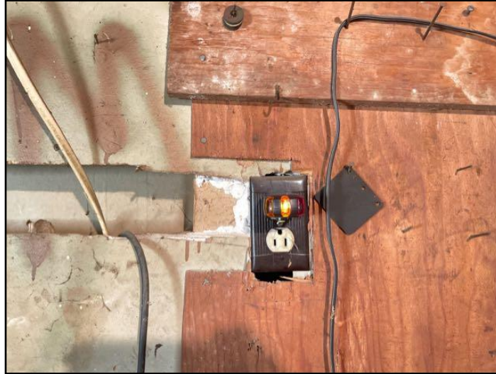
41. Three Prong Outlets Tested Open Ground
