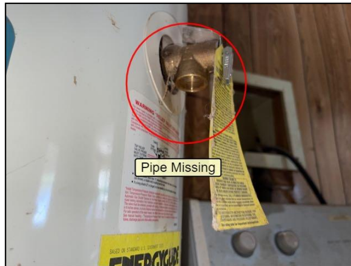
60. Discharge tube missing
